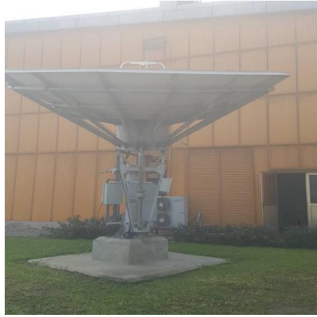
New VSAT at Kinshasa Ndjili
